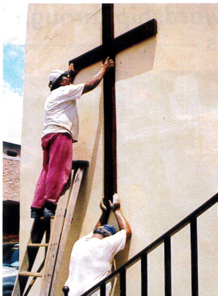
Construction workers Don Pablo (bottom) and his son Jorge (on ladder) hanging the cross for the new seminary building in Mexico. On the day the seminary was dedicated, Israel Rodriguez graduated, raising the number of national pastors in Mexico to five.
