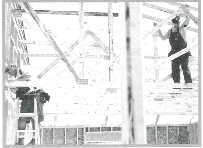
Members of Builders For Christ (BFC) helped St. Matthew, Port Washington, Wis., build their church in 1998. BFC provides volunteers to help build facilities at reduced cost.
