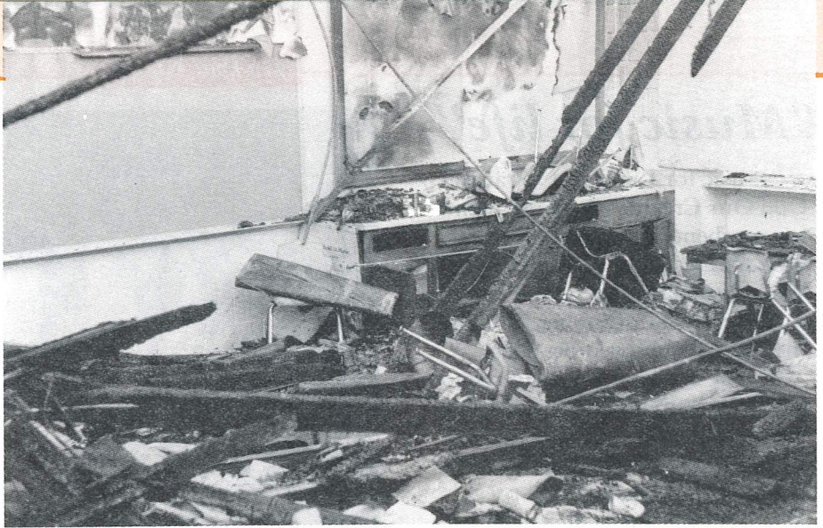
Fire damage at Christ the Lord
