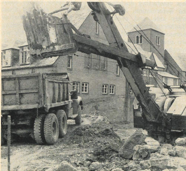
Excavating for the Library Building at Wisconsin Lutheran Seminary. The north wall of the chapel wing is seen beyond the truck.
