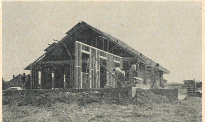
THE EDUCATIONAL WING was framed in and the framework of the church proper was begun when this picture was taken (Calvary, Dallas).
