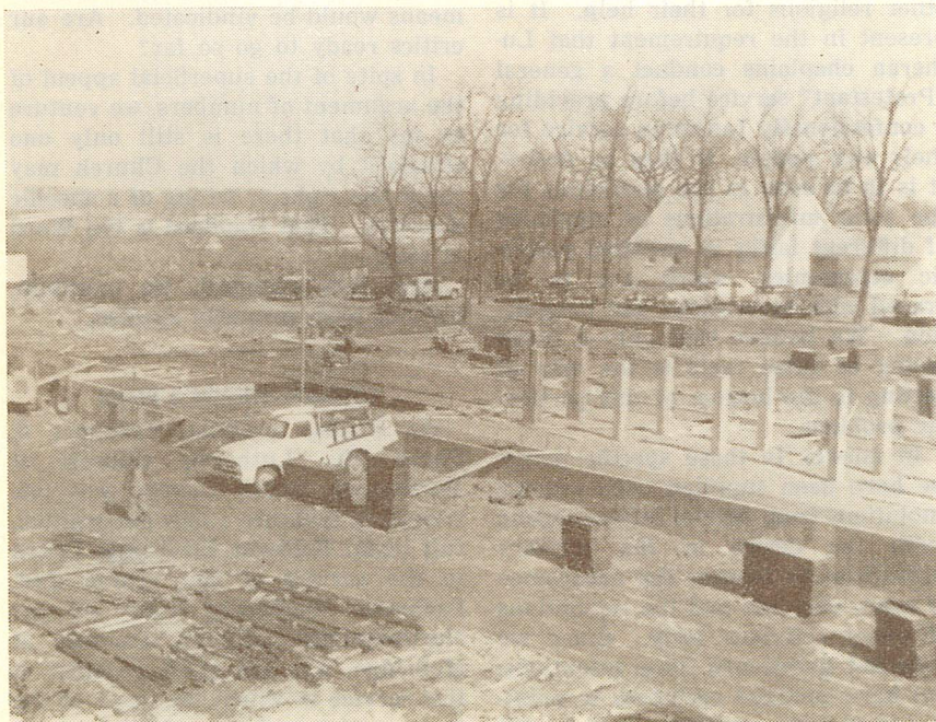
The foundation is laid for the new dormitory at Northwestern College. In the background is a view of one of the new professorages.
